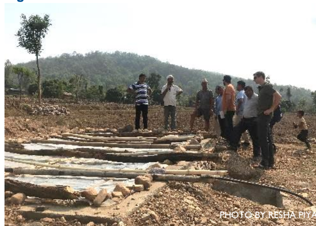
Figure 9: Hamtad soil cement tank and offtake
